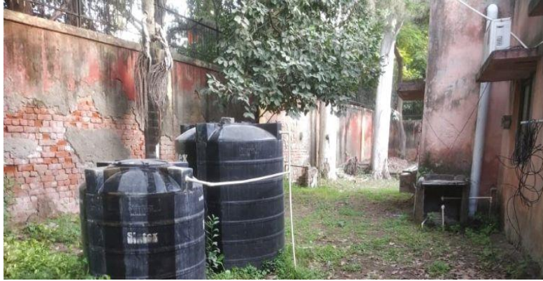
Figure : Water storage sites in college campus
